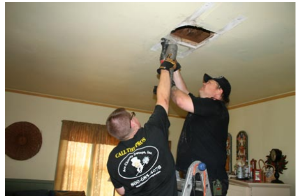
Skip and Tyler Cresswell prepare the ceiling for the new stove pipe and venting system installation
