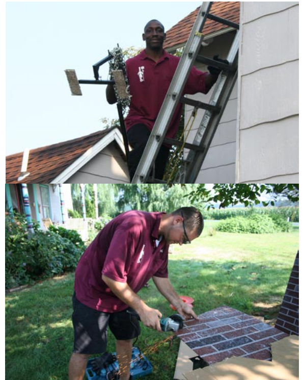
Colby Hostedler prepares the chimney surround as Lawrence Green prepares for its installation.
